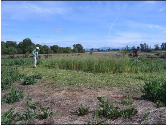
Weed whackers were used instead of mowers to clear vegetation from new tarp sites. The mower was unable to get close enough to the ground and remaining stems could puncture the tarp.
